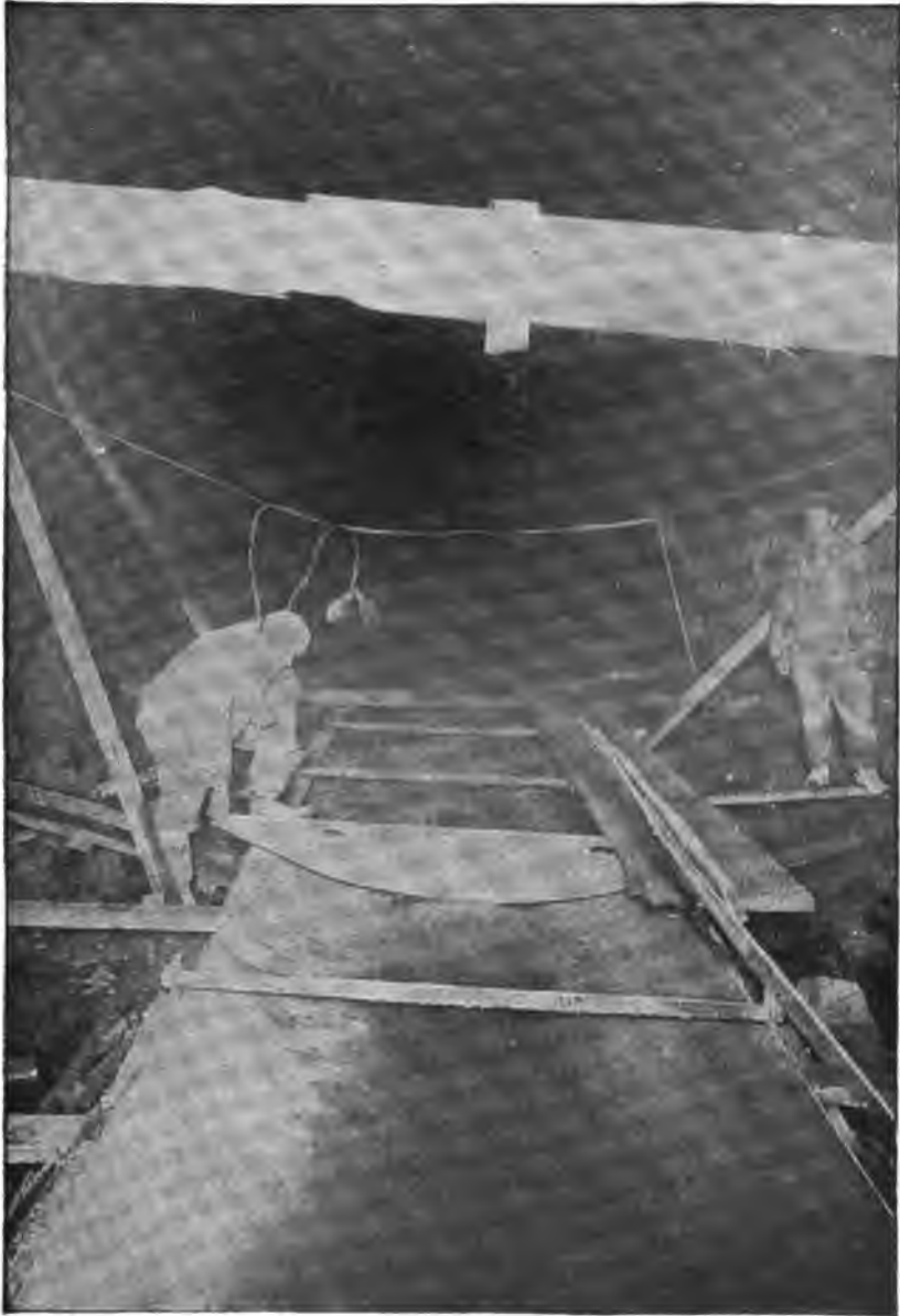
PLATE 99. —Screeding Invert for Rondout Siphon. Concrete was laid between continuous forms held in position by pipe spreaders. Skip is 5 feet wide with radial side joints and bonding grooves.
